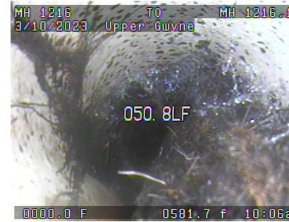
< A picture of a sewer lateral connection with heavy root intrusion at the 6" to 4" Transition, as viewed from the Lateral Launch Camera.
