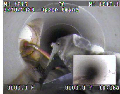
< Image from a Lateral Launch CCTV Camera System. Taken from the camera view of the "Tractor" which has driven to a lateral connection point in the sewer mainline, visible coming in from the left side. The orange cable extending from the tractor contains the launch camera, to inspect up the line (Visible in the PIP at the bottom right).
