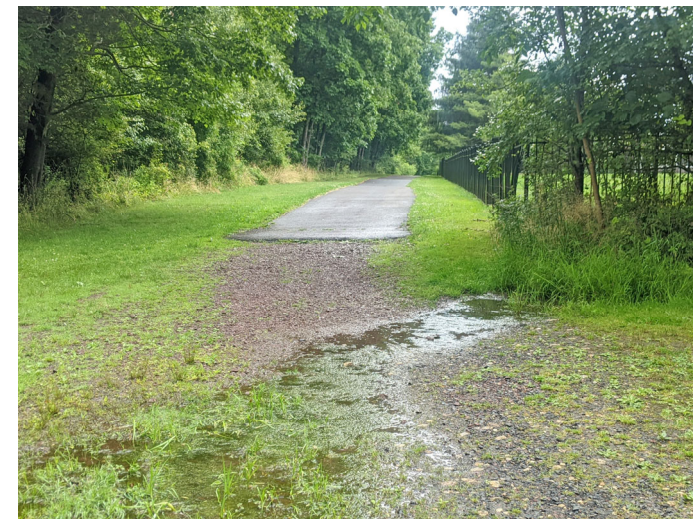
Survey respondents requested that a solution be found to correct ongoing drainage problems along the existing shared-use path between West Point Pike and Parkside Place
