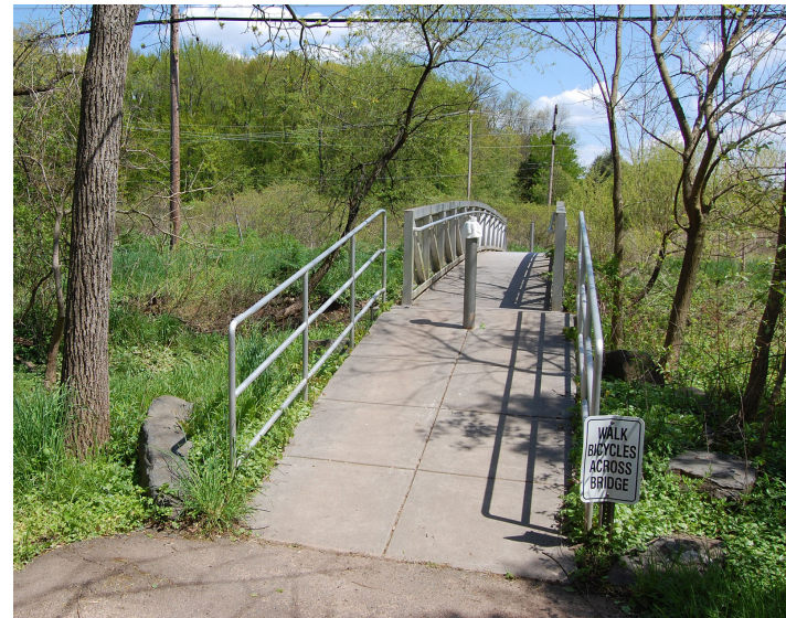
Existing trail bridge over Wissahickon Creek between West Point Pike and Parkside Place
