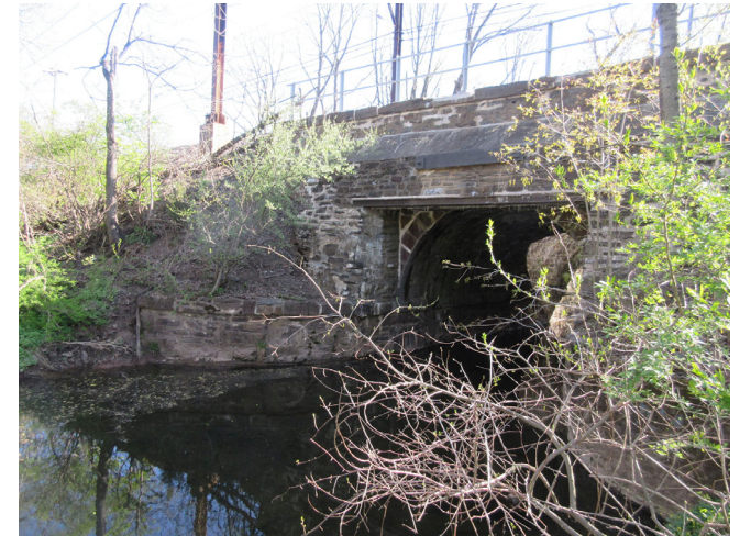
The existing stone arch beneath the SEPTA Lansdale-Doylestown line cannot accommodate a shared-use path
